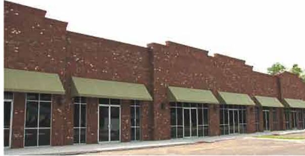
St. Laurent Properties New Commercial/Retail Construction 480 South Ronald Reagan Blvd. Status: Under Construction
